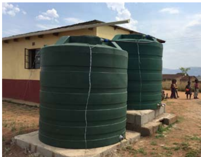
NCP with 2 tanks
